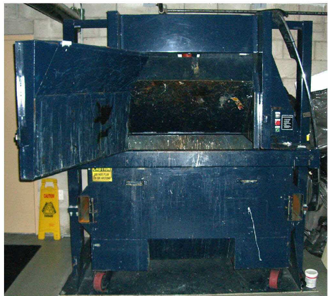
Each Garbage & Recycle Room contains a 3-cubic-yard Trash compactor capable of compressing 9 cubic yards of household trash.
